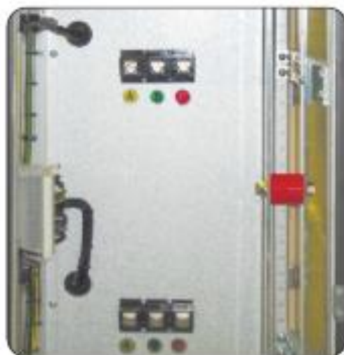
Incoming and Outgoing Line on the side
