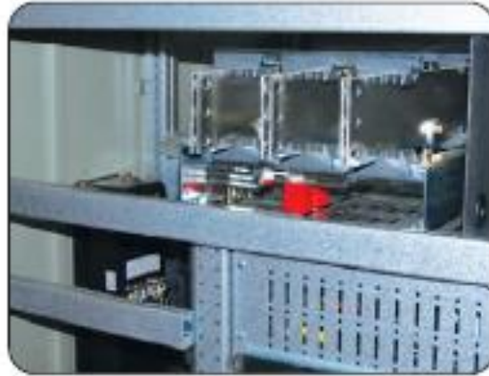
a) Horizontal Buses on the Top of the Cabinet
