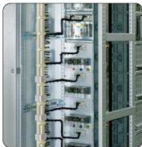
Incoming and Outgoing Line at the back
